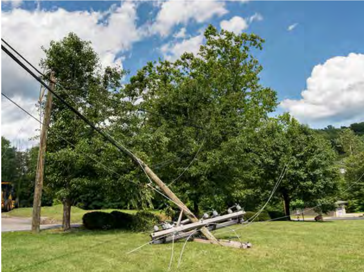
A downed power line following a storm. In the fall of 2011, nearly a quarter of a million Southern California Edison customers were without power after a windstorm toppled utility poles.
