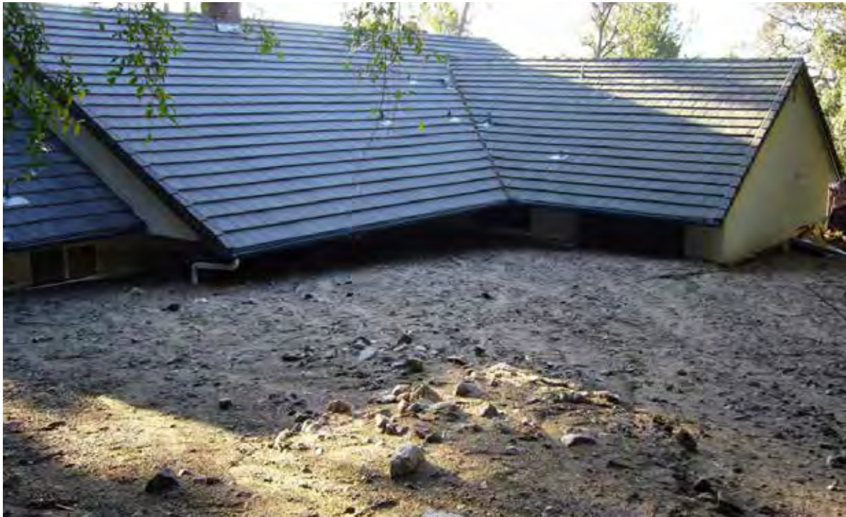
A home west of Briar Wood Canyon is engulfed in post-fire debris flow from a rainstorm following the Station Fire. Photo credit: Susan Cannon, USGS.
